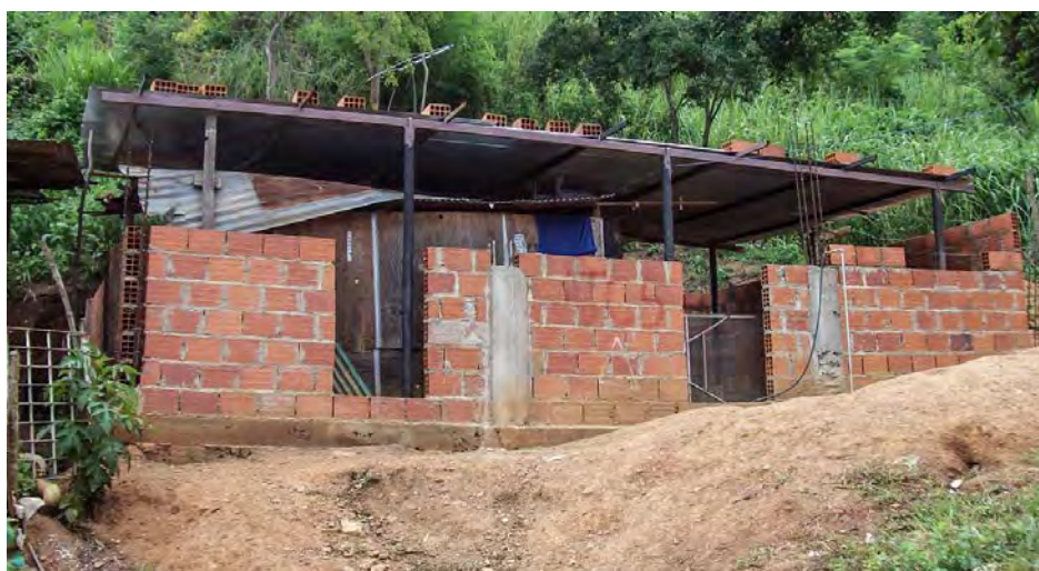
Picture 4. Progressive construction technique in order to add environments and improve the structure quality
