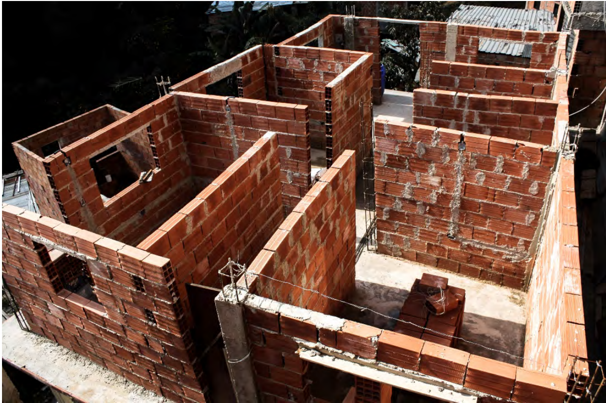
Picture 6. Building the second floor of a house with advanced structure living configuration
