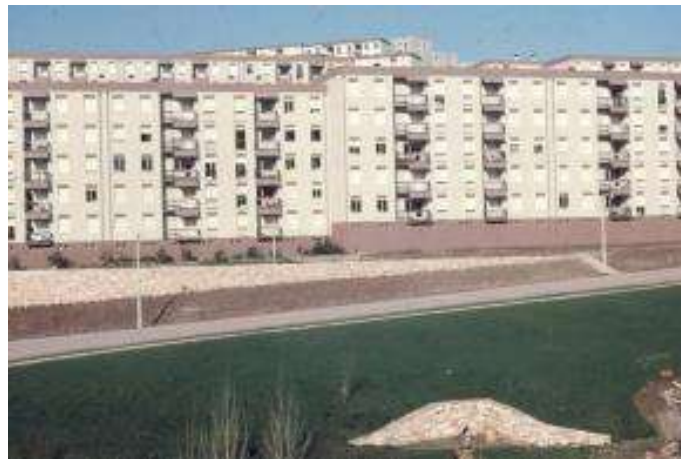
Figure 47. Assembly of the heavy panels on site and view of the first completed buildings
