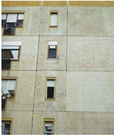
Figure 60. SAC: Micro-fissures in exterior panels
