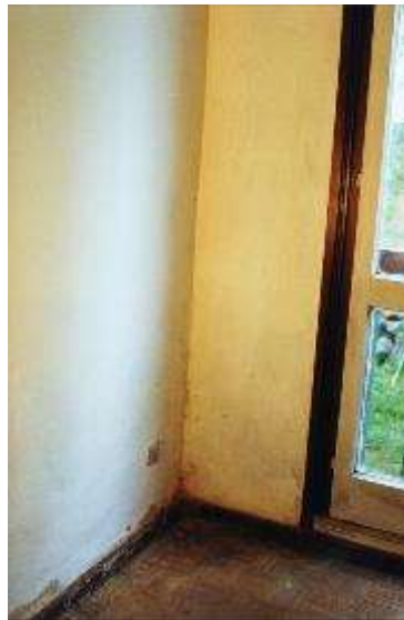
Figure 61. QM: Interior humidity coming from exterior panels, caused by the incorrect assembly of the panels or by the lack of compression in the sealants of the panels' joints
