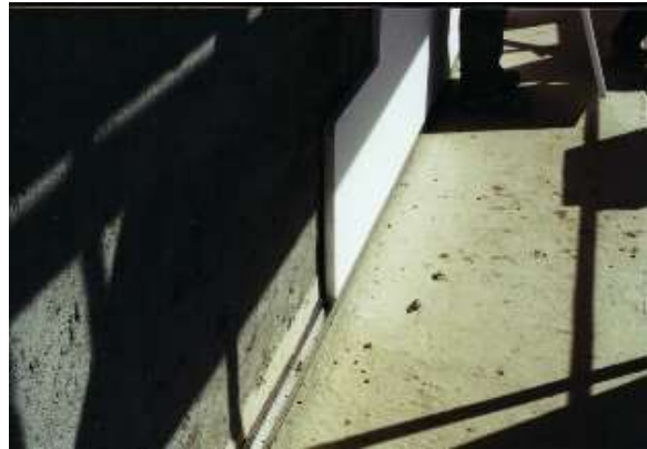
Figure 66. Building work in progress (Science Faculty of Lisbon Building) – Special fitting profiles to allow an adequate fitting of the pieces and better continuity
