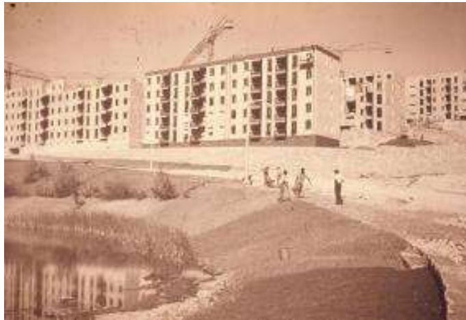
Figure 46. Assembly of the heavy panels on site and view of the first completed buildings
