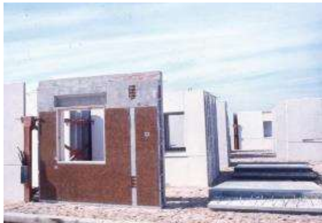
Figure 31. Storage area of the exterior panels and prefabricated elements (interior panels) storage yard
