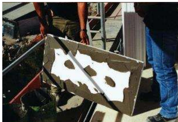
Figure 65. Building work in progress (Science Faculty of Lisbon Building) – The insulation board with adhesive coat applied with points and bands
