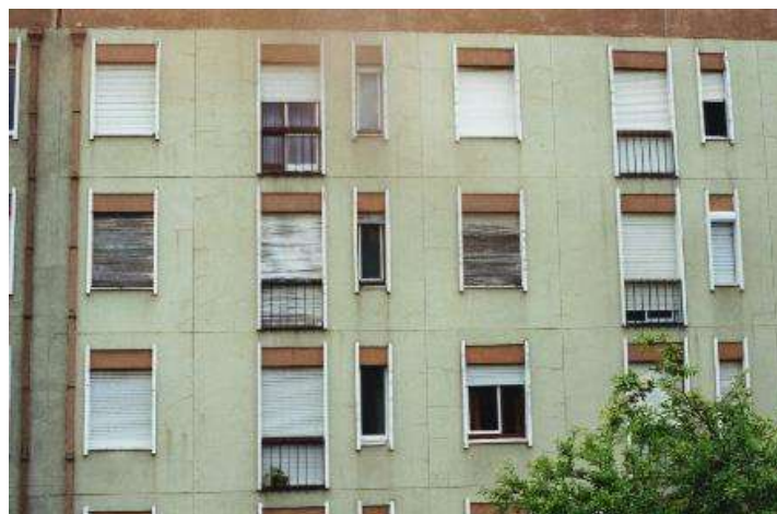
Figure 59. SAC: fissures detected in the external surface of the outside panels
