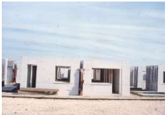
Figure 32. Storage area of the exterior panels and prefabricated elements (interior panels) storage yard
