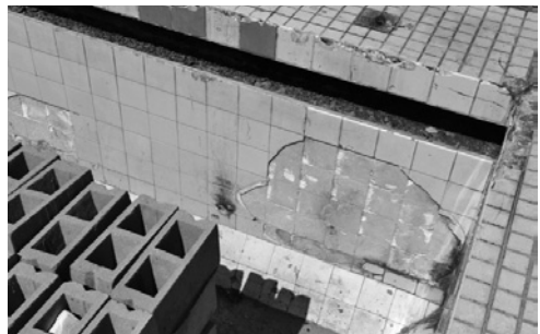
Fig. 8 – Autophagy, or how the foundations of the Hotel swimming pool feed the production of bricks. Colour figure available online.
