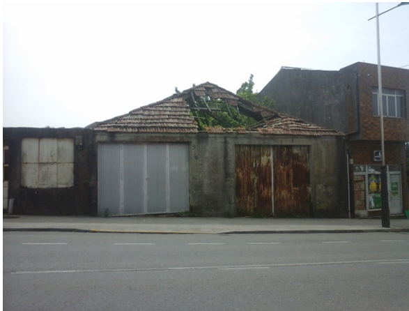
Fig. 6 – House converted into a garage, currently in ruins, Santa Comba, May 2015. Colour figure available online.
