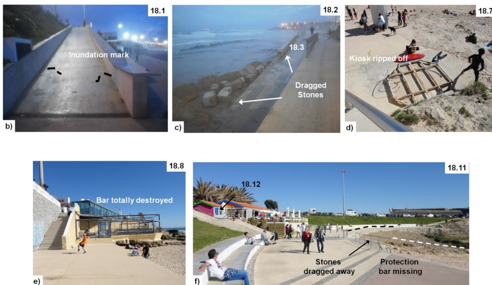
Fig. 8 – Field survey at Carcavelos beach: a) Framework; b) Inundation mark; c) Stones from the ramp were dragged away; d) Kiosk ripped away; e) Restaurant completely destroyed; f) Point 18.12 shows the maximum inundation area.
