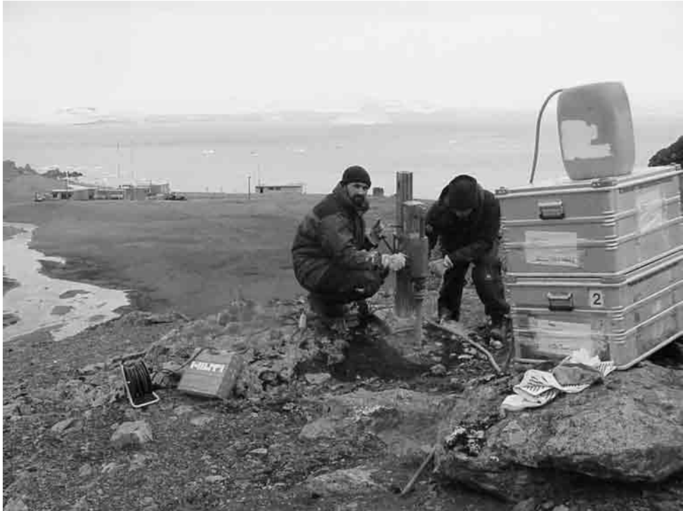
Fig. 1 – Shallow borehole drilling for active layer monitoring at Incinerador site in Livingston island in January 2000.
