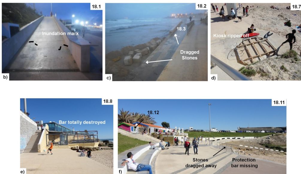
Fig. 8 – Field survey at Carcavelos beach: a) Framework; b) Inundation mark; c) Stones from the ramp were dragged away; d) Kiosk ripped away; e) Restaurant completely destroyed; f) Point 18.12 shows the maximum inundation area.
